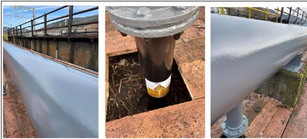
Figure 17 - Photograph showing the condition of the newly refurbished crossing and new warning stickers
