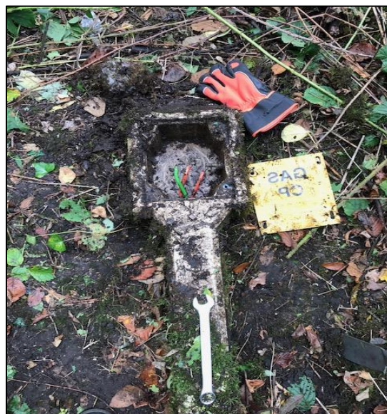
Figure 12 - Test Post in poor condition
