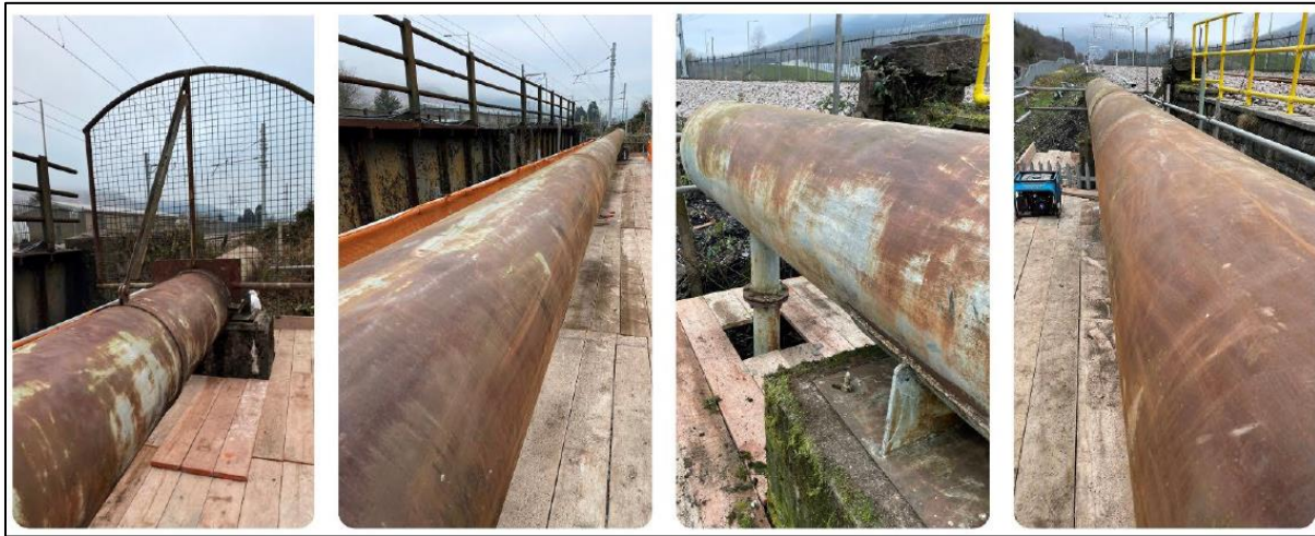
Figure 16 - Photographs of the poor condition of the crossing prior to refurbishment
