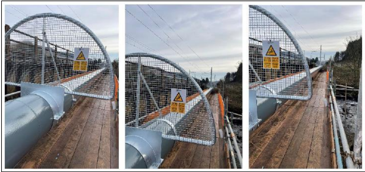
Figure 18 - Photograph showing newly installed crossing guards with warning stickers
