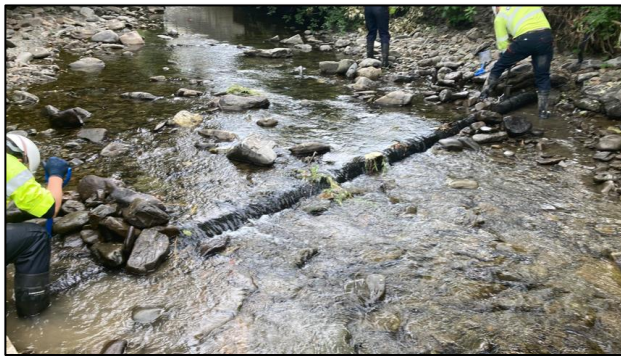
Figure 20 - Exposed IP main
