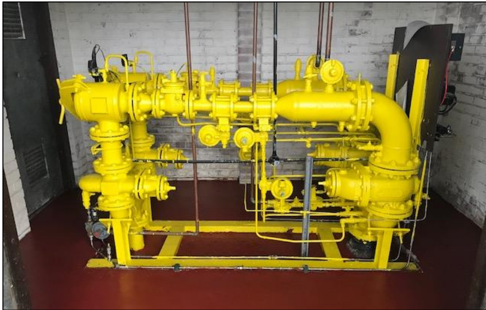
Figure 1 - Example of Governor Installation
